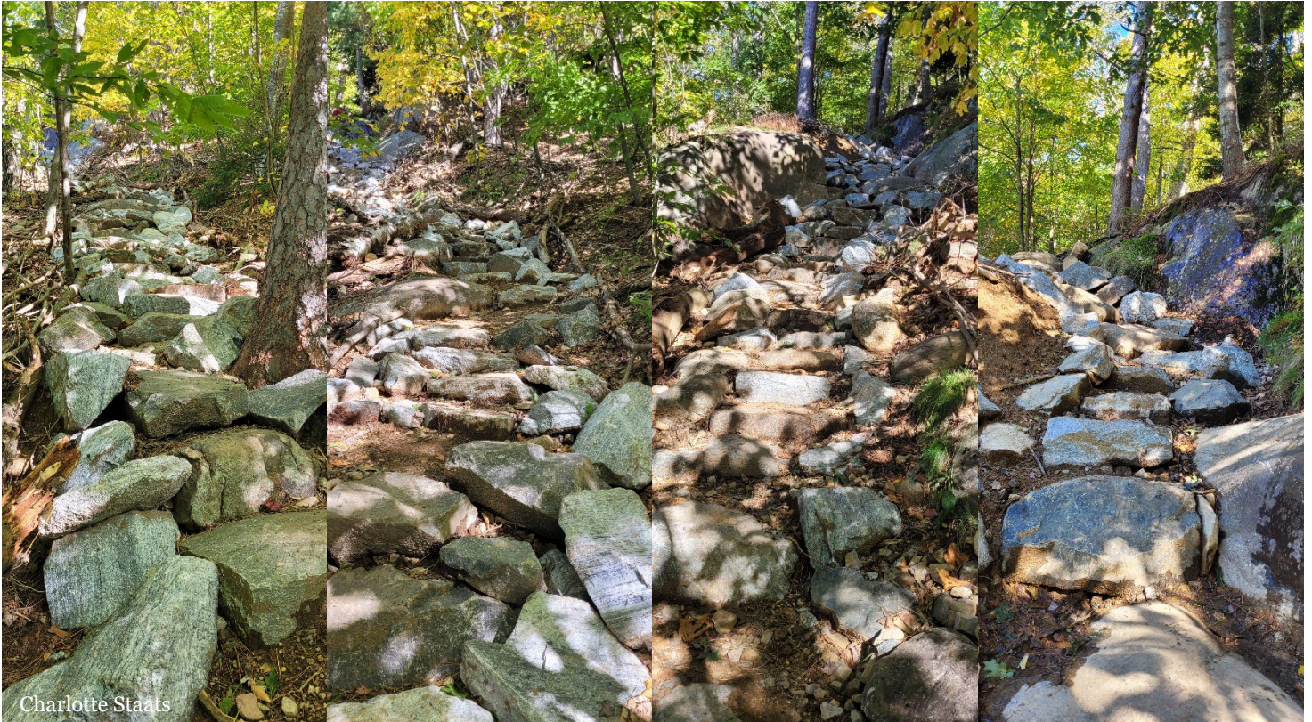
A series of photos of the rock staircase built on Poke-O-Moonshine this year. Left to right: the bottom of the staircase, two middle portions, and the top of the staircase.
